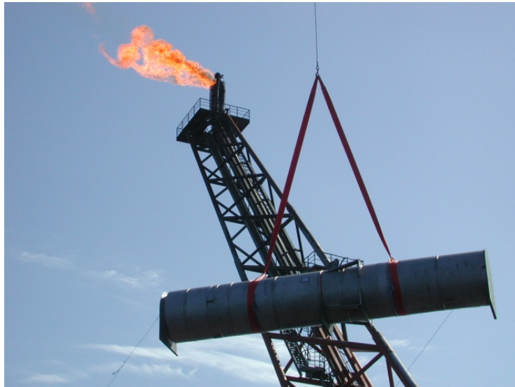
BP Valhall – new exhaust stack
