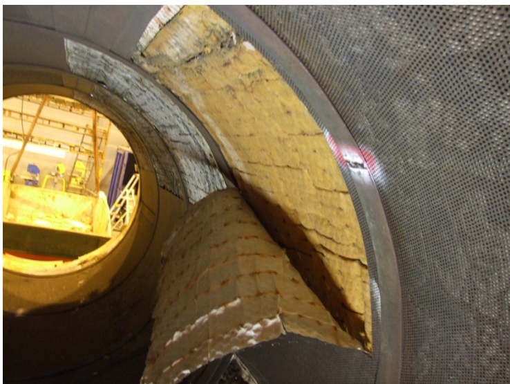
Visund 4 tr. exhaust stack - post-mortem examination at our workshop
